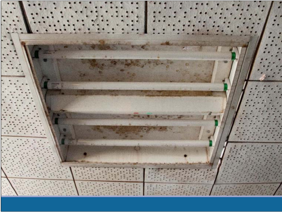
Examples of facility needs: leaky roofs at many schools.
